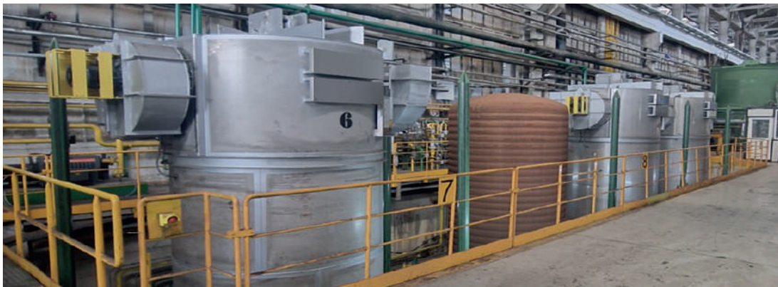
New bell annealing facility - Copper segment
